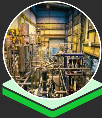
Research Pilot Plant
